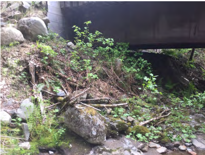
No riprap in front of left abutment
